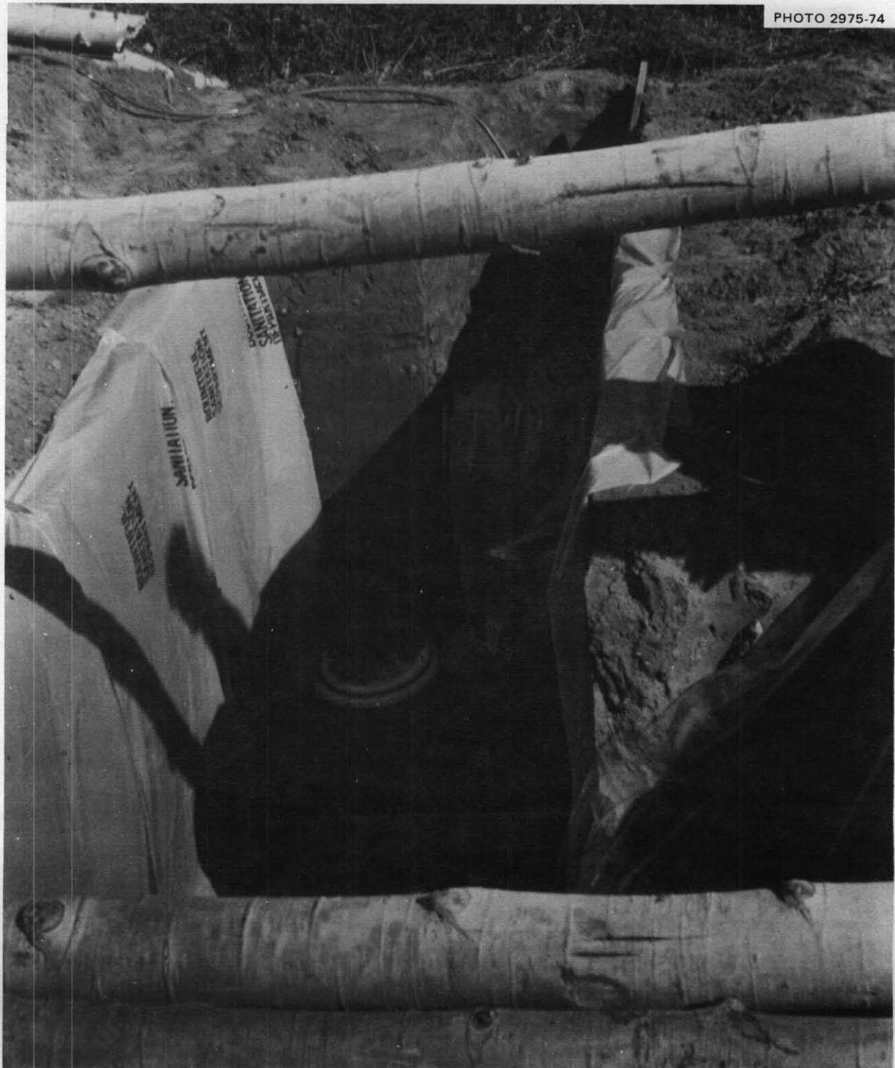
Fig. 4.6. Covering the main trench with 9-ft aspen logs. These logs were 4 to 6 in. in diameter at their small ends – thus being stronger than necessary to support the planned 3 ft of earth cover.
